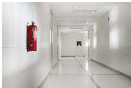
Figure 3. Fire extinguisher installed in a building
