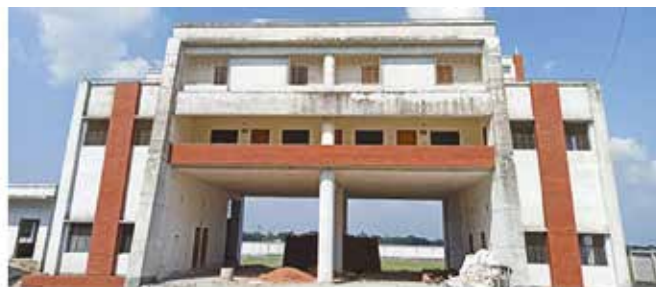
Figure 4. Construction of a fire service and civil defense unit on BAU campus after the 2018 fire
