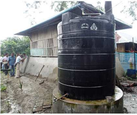
Figure 1. Water tank for rainwater harvesting.
